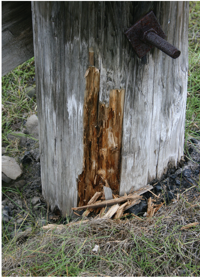
Figure 13. Detail showing rot in the wooden pole of a cable car buck in Longyearbyen, Svalbard. Source: Anne-Cathrine Flyen, reproduced with permission.
