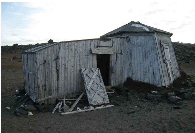
Figure 1. A trapper's cabin built in 1904 by Norwegian trappers at Kapp Lee, Edge Island in Svalbard. The picture was taken prior to restoration of the hut in 2009 by the Governor of Svalbard. Source: Anne-Cathrine Flyen, reproduced with permission.
