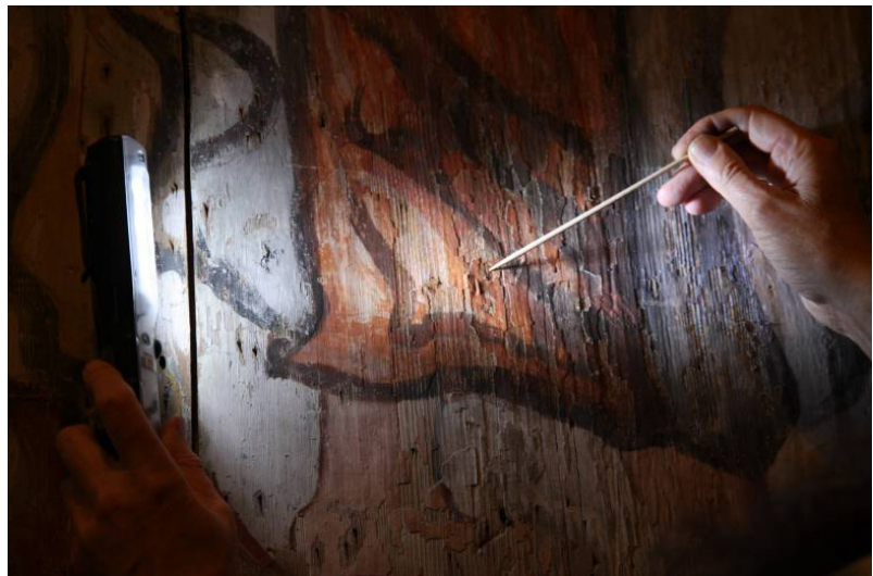
Figure 8: Flaking paint on the north wall in the chancel of Heddal stave church. Photo: Mille Stein, NIKU, 2013.
