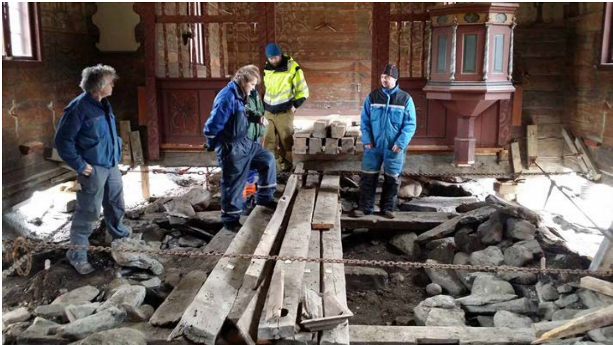
Image 6 Checking the conditions under the floor. A lot of sludge and moisture had accumulated here. Photo: Monica Finden, Aurland kommune
