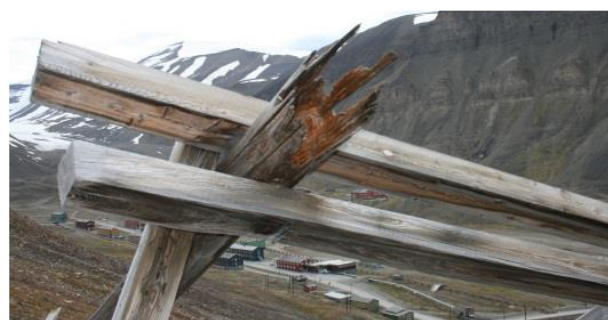
Fig. 8. Characteristic pattern of extensive, internal fungal decay in wood with soil contact at Longyearbyen, Svalbard. The external layer of wood is undamaged, whilst the inner parts are heavily decomposed. Photo: NIKU v/A.C. Flyen.
