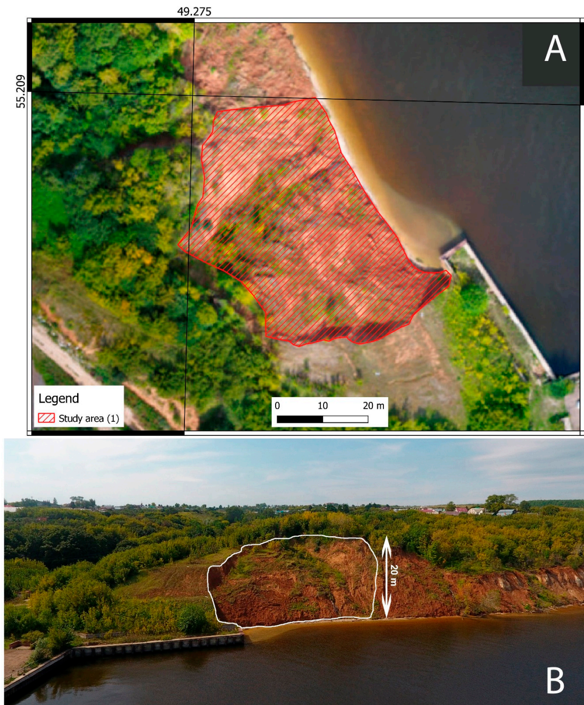
Figure 2. Aerial (2019) (A) and oblique views (B) of the shoreline and the landslide body at Site 1.
