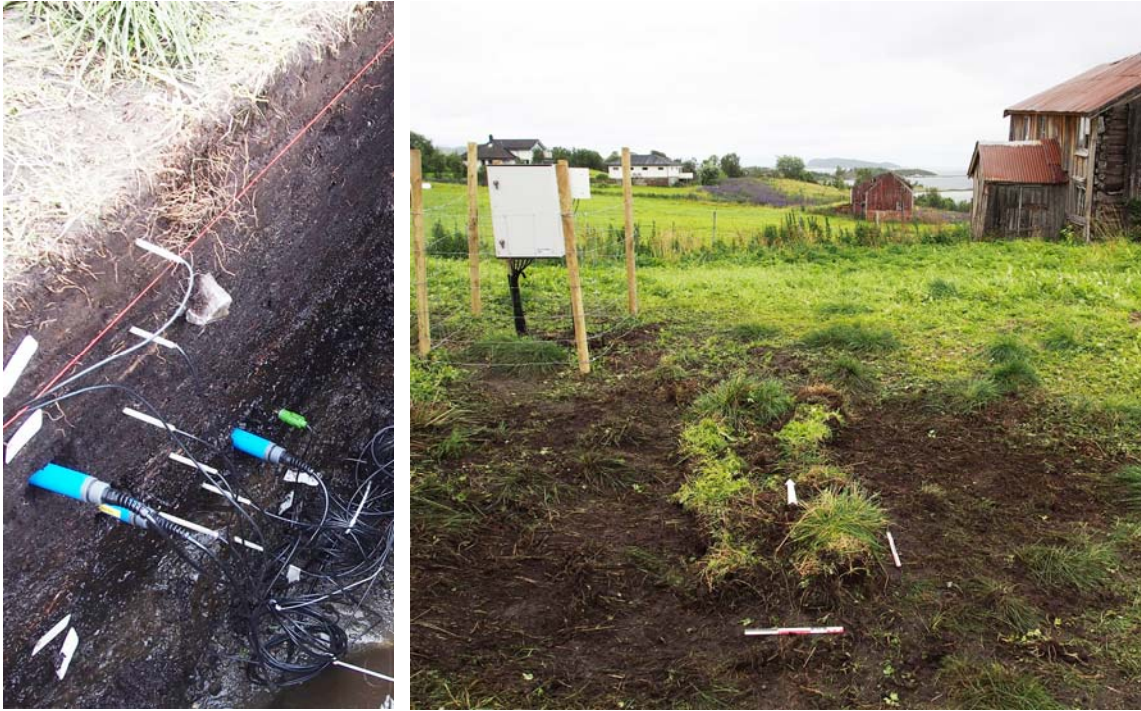
Figure 23 Monitoring equipment installed. VVM/NIKU (left).
