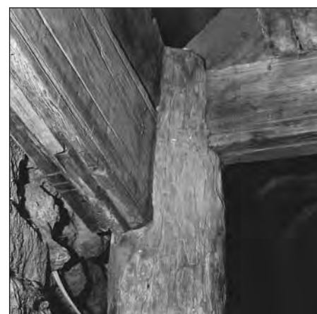
Figure 15. Post, cross beam and head beam in the dwelling room of the farm Keldur in Iceland. Note the groove from a stave wall and the decorative mouldings on the beams.
